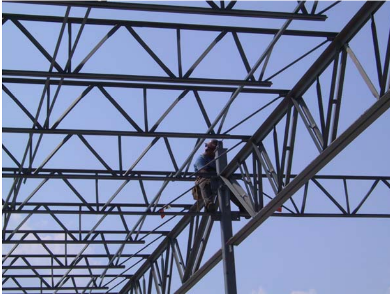
Figure 12 Column joist being connected; Bottom chord is “knifed in” between vertical stabilizer plate
