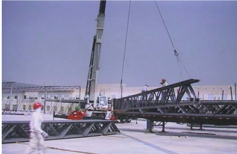
Figure 4 Lifting with a crane using two chokers configured in a basket hitch and two-way spreaders
