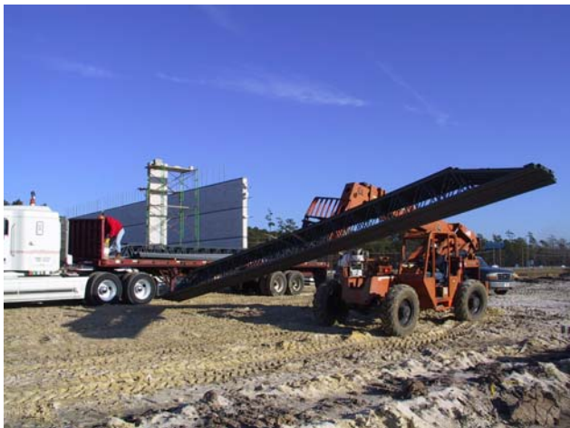
Figure 7 Improper joist handling – Load is not balanced on forks
