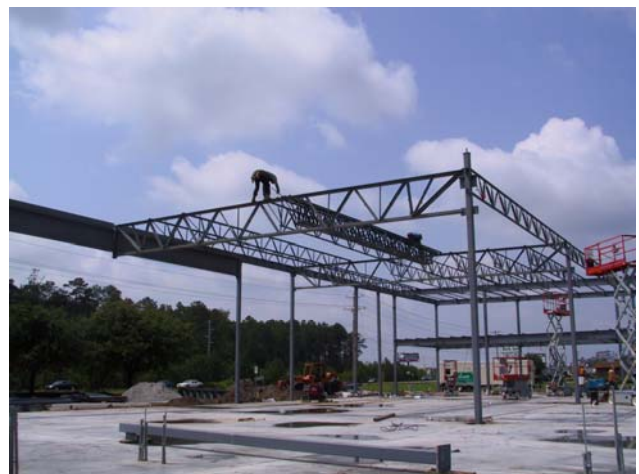
Figure 15 Shortspan joists being spread out along Joist Girder top chord by two Erectors
