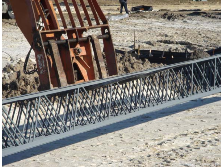
Figure 9 Proper joist handling - Forks have solid contact with joist chords and therefore do not put unnecessary pressure on web members
