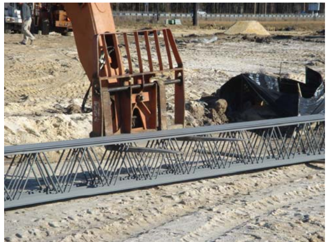
Figure 8 Improper joist handling – Fork on left is wedged between two web members, could damage webs
