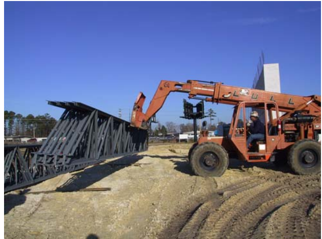
Figure 6 Storing a bundle of Joist Girders with a fork type lift on proper timbers
